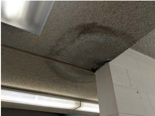
Water damage asbestos ceiling
